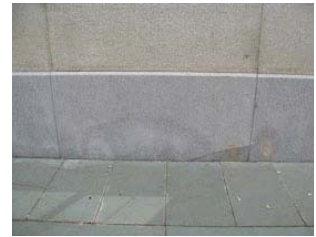
CRACKING AT GRANITE BASE, WEST COURTYARD
