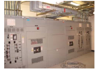
ELECTRICAL DISTRIBUTION EQUIPMENT
