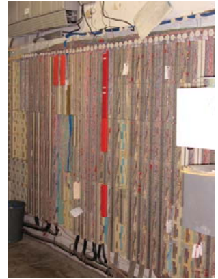
BASEMENT TELEPHONE ROOM
