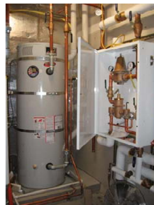
WATER HEATING SYSTEM
