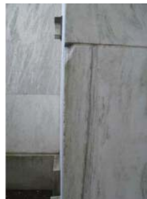
EXAMPLE OF SPALLING AT THE CORNER OF A MARBLE PANEL
