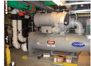
WATER CHILLER CH-1
