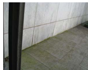
BIOLOGICAL GROWTH AT SLATE PAVERS AND BASE OF BUILDING
