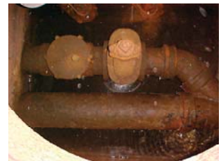
FLOODED WASTE PIPING VAULT
