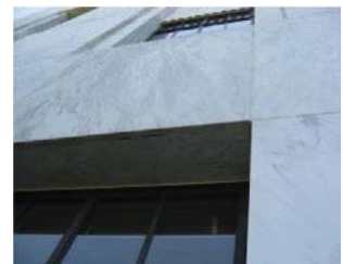
EXAMPLE OF CRACKING AT THE UNDERSIDE OF THE WINDOW HEAD
