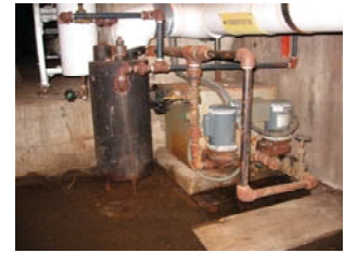
CONDENSATE PUMPING STATION
