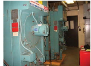
HIGH PRESSURE STEAM BOILERS
