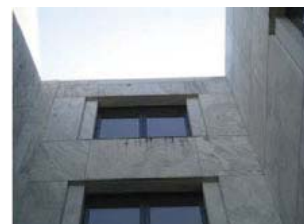
INSTANCE OF SOILING AT THE WINDOW SILL
