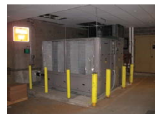
PROCESS WATER CHILLER
