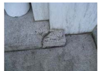
CRACK AT TOP TREAD, STAIRS ON WEST ELEVATION
