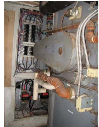
POOR PANEL ACCESS
