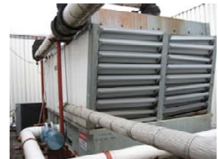
COOLING TOWER CT-2
