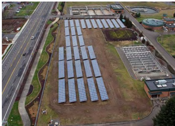
Photo 5: The 419 kW DC PV array at the City of Gresham Waste Water Treatment Plant, which is currently the largest ground-mounted installed solar array in Oregon.
