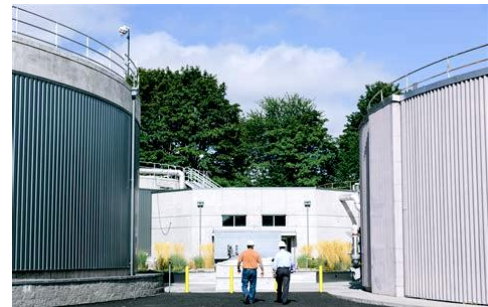
Anaerobic digesters at Oregon’s first RNG project: Columbia Boulevard Wastewater Treatment Plant in Portland, OR.
