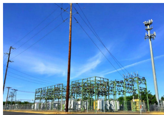
Substation in Canby, Oregon.
