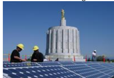
Figure 2. Solar Panels on Oregon State Capitol
